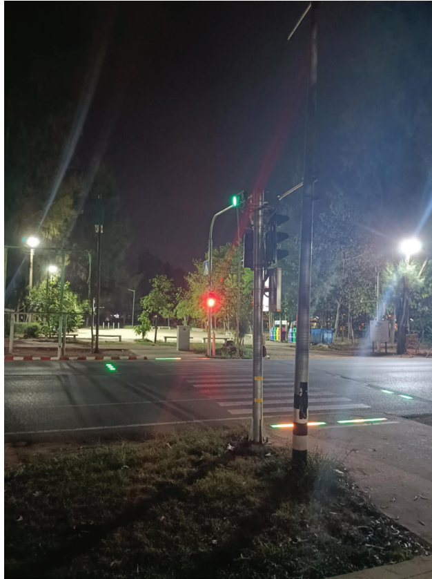
Figure 8 Pedestrian Crossing LED Lighting in Khon Kaen University, Thailand
